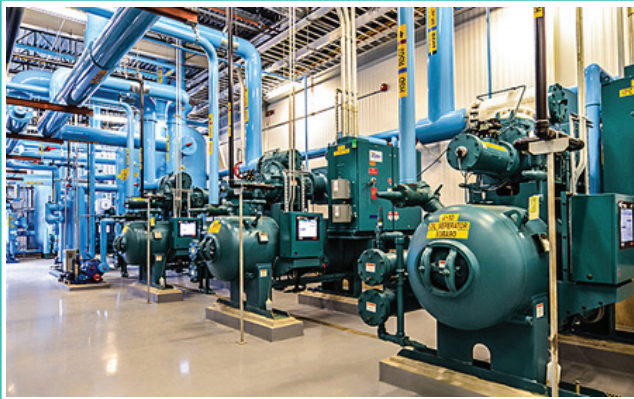
Figure 4: Well-designed and maintained refrigeration plant
